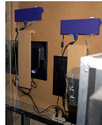
Roku installation of Video switching exhibit
